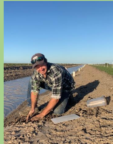
Two V drains were construction for retention of water next to the tree lines
